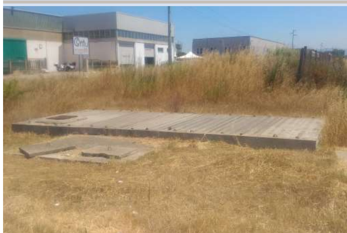
Vasca interrata in c.a.
