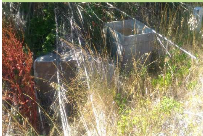
Vasca in fibrocemento
